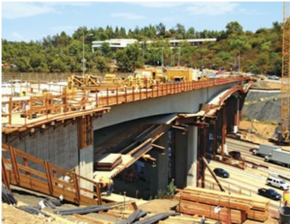
Photo by Greg Aragon for ENR Demolition of a bridge is one milestone in a busy time for Metro construction.
